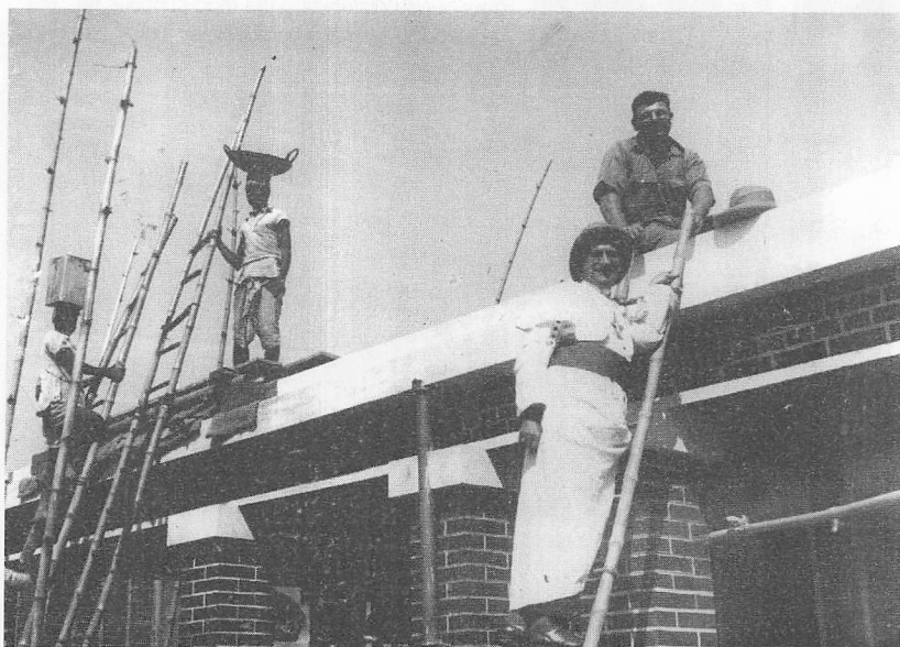
St. Joseph's Dispensary near the Cathedral under construction. Bro. Charles Castelli who worked with Father Bishop for many years as an architect in Krishnagar diocese is seen on the terrace.
